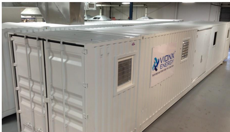
VionX Energy has installed a large-scale vanadium flow battery storage system to the U.S. Army at Fort Devens.
